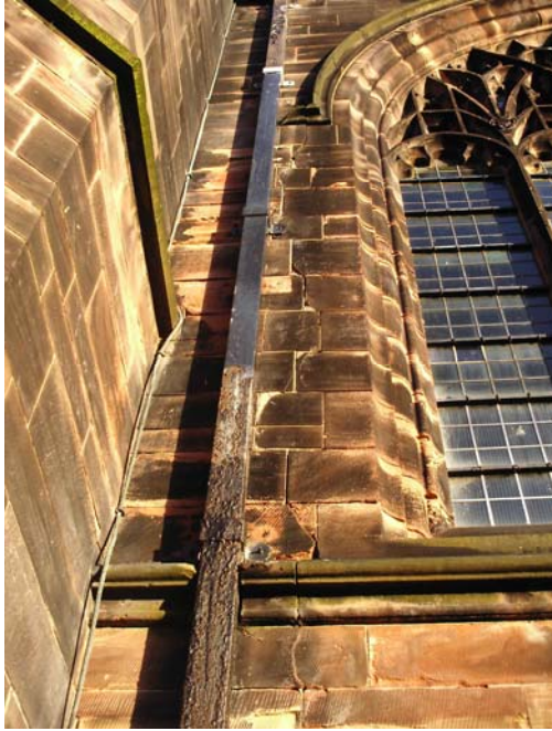
Fig. 12.12 Damaged masonry caused by defective rainwater pipe
