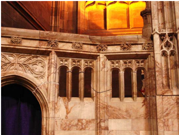
Fig. 12.11 Detail of damage to reredos
