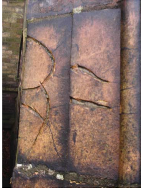
Fig. 5.22 Detail of terracotta coping, note that cracks appear to have been ground and cement filled previously, as a holding repair
