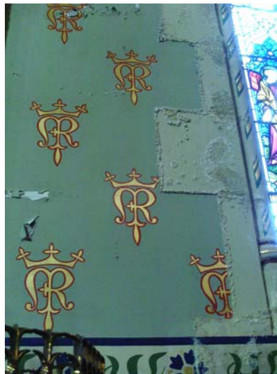
Fig. 8.16 Water damaged wall decoration, 2005
