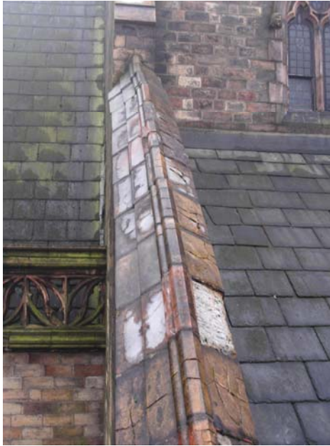
Fig. 5.21 The existing terracotta copings, to be renewed
