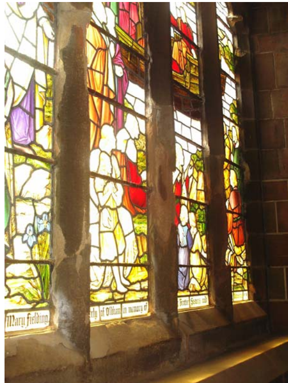
Detail of salt damaged tracery
